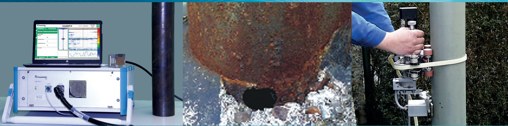
Left: LIMAtest® inspection system; right: Corrosion below soil level
